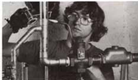
Air purger, valves and copper pipes were plumbed and soldered according to the manufacturer's recommendations.
