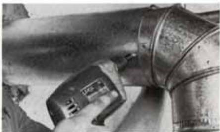
Flue pipe sections were fastened at all joints with sheet-metal screws to keep them from separating due to vibration.
