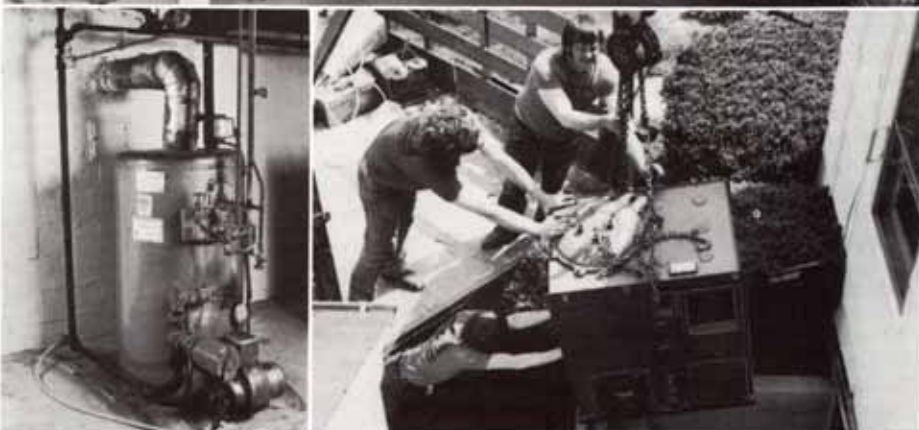
Multifuel unit (top) operates at efficiency of 84 percent (oil) or 62 percent (wood). Old oil burner (below, left) was 68 percent efficient. Door and unit sizes were compared before boiler was delivered. Basement entry eased task of getting new unit in, old one out.
