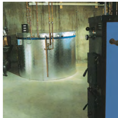
Excel boiler with Storage Tank.
