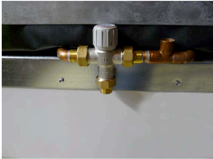
Domestic water exchanger installed
